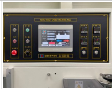
Touch Panel Controller
